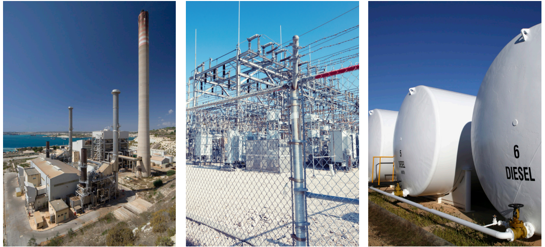
Figure 9: Power plants, electrical sub-stations and fuel tanks are some of the application areas for Axis temperature alarm cameras.
